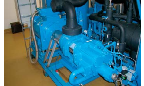
Ethyleneglycol Chiller Unit
